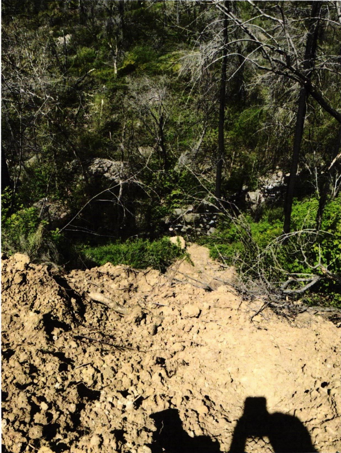
Figure 4: Sidecast sediment from road discharged to stream channel below.
